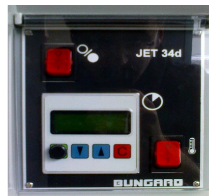
Control panel with new timer
